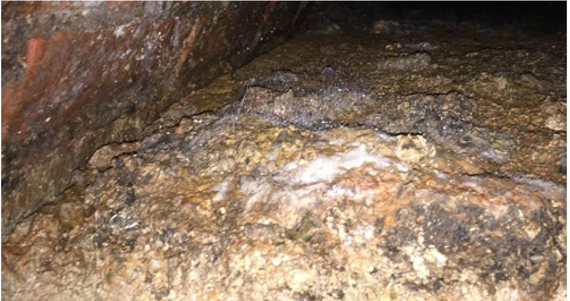
Fatberg blocking a sewer in Cardiff
