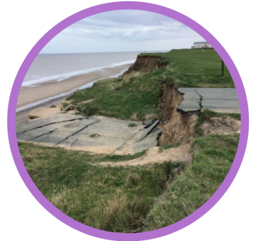
Road collapse near Aldbrough © Michael Livsey
